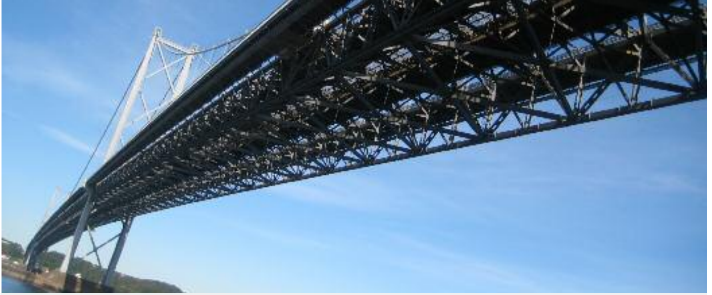
The Forth Road Bridge, built in 1964 with Scottish steel. No Scottish or British steel will be used in the new Queensferry Crossing.
